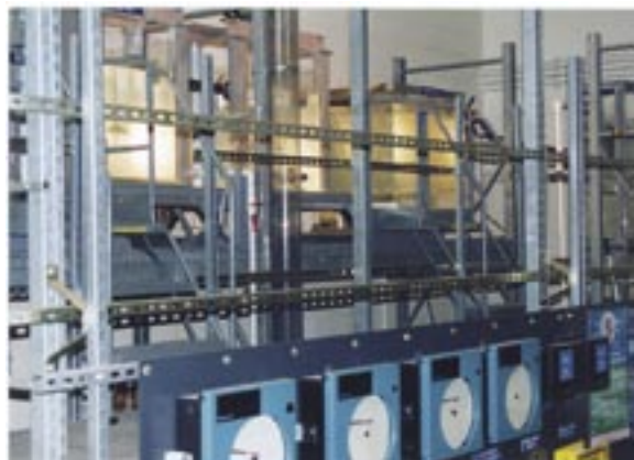
The pilot size water filtration and purification system at the Environmental Training Center (ETC)
